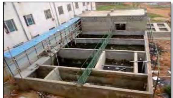
1000kld STP within the campus
