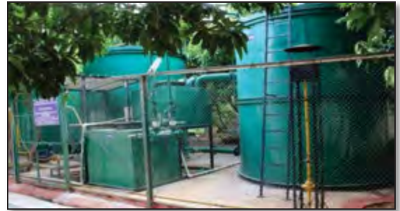
Biogas plant within the campus
