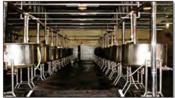
Steam based Mechanized kitchen
